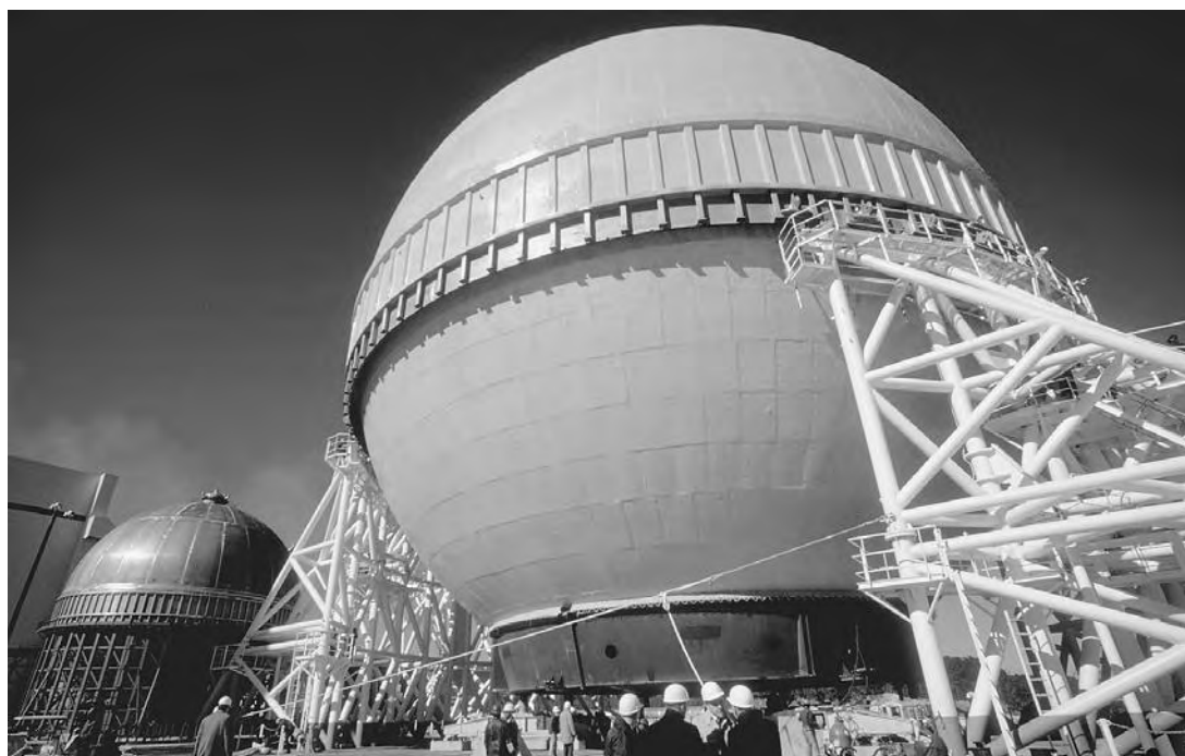
THIS HUGE LIQUEFIED NATURAL GAS CONTAINER WILL BE INSTALLED ON A SHIP. THE VOLUME OF THE LIQUEFIED GAS IS FAR LESS THAN IT WOULD BE IF THE GAS WERE IN A VAPORIZED STATE, THUS ENABLING EASE AND ECONOMY IN TRANSPORT. (Photograph by James L. Amos/Corbis. Reproduced by permission.)
